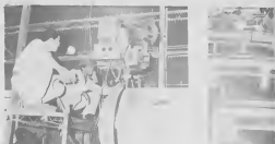
M. Werleman and E. Rummel, welding the head of a bundle shell with an automatic submerged welding machine.
